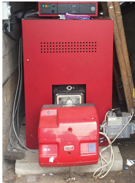
Natural gas boiler and burner
