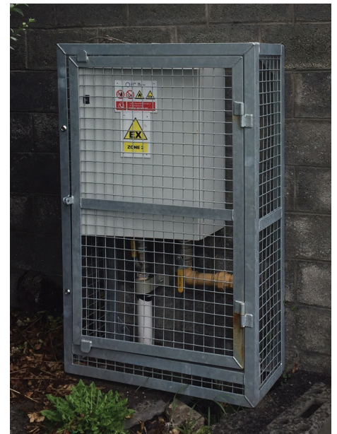
Natural gas meter with meter protection
